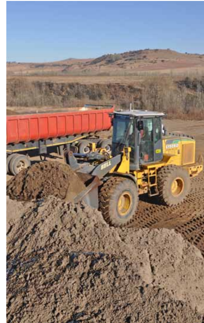
A Bell L1506D Front End Loader was the first new piece of equipment bought by Bethlehem Sand & Klip back in 2006. Today the machine is still a strong and reliable part of the fleet and is used extensively for loading products onto the company's interlinked and rigid tipper fleet.
