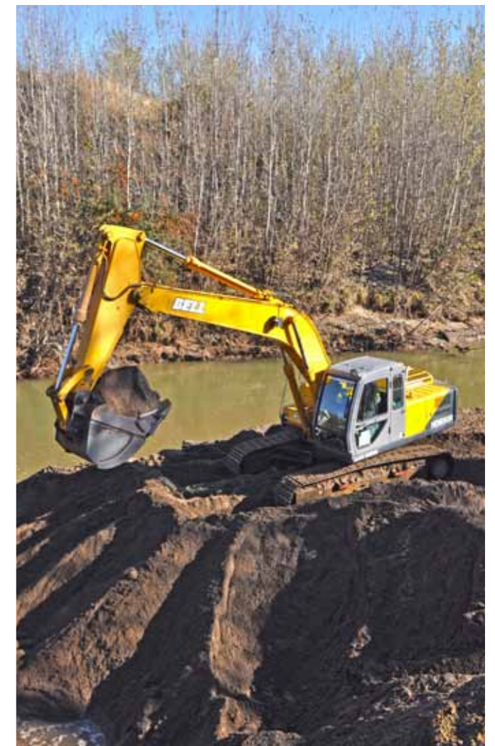
Bethlehem Sand & Klip took delivery of a new Bell HD820E Excavator just over a year ago and the machine sits at the heart of the company's sand-mining operation, able to build stockpiles with ease.
