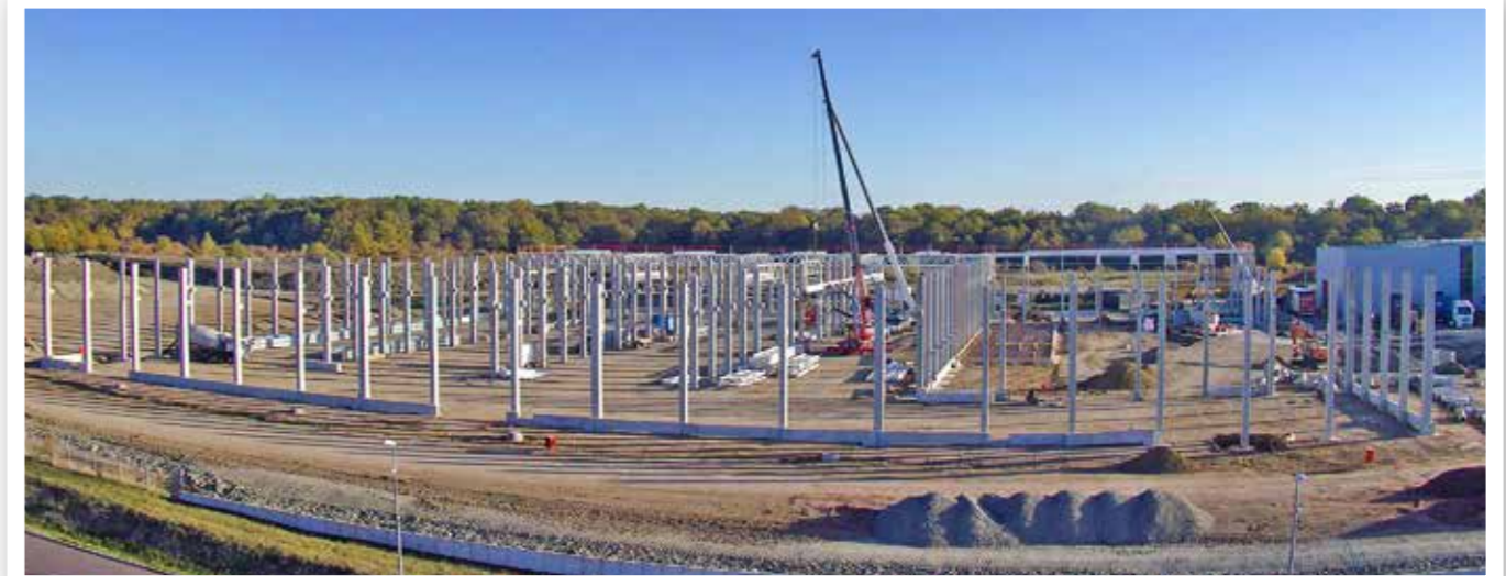
The new 12 000m 2 factory extension at the Bell ADT plant in Eisenach-Kindel will be operational in mid-2019.
